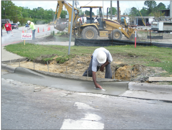
A curb ramp on a section of the rail trail being installed at Marine Blvd. and Bell Fork Road.
